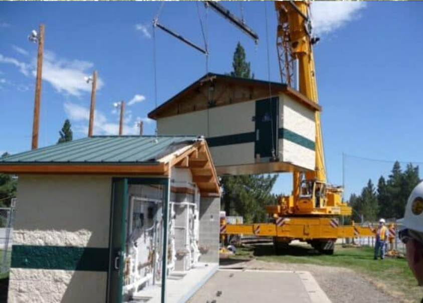
Costly to Install
