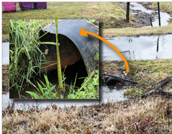
Figure 25. Existing culvert under 41st Street trail. Areas is near Northwest Branch trail intersection.
