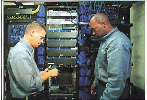
Johnson Controls Employs the Best Trained Service Personnel in the Industry.
